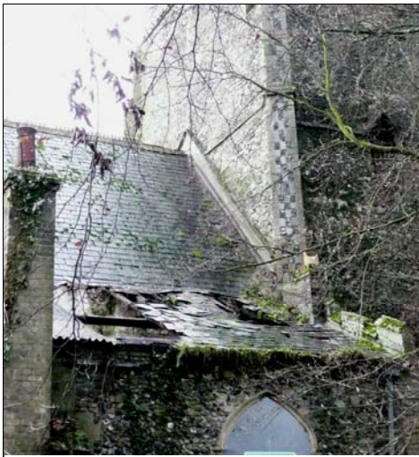
The roof of the north aisle/vestry of St Mary the Less, which needs repairs.
